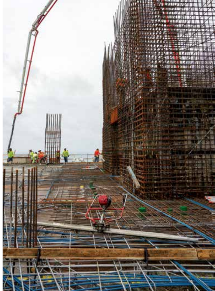
Despite working over rebar from one of the structure's cores, the placing booms were able to access all parts of each 25,000-square-foot floor.
