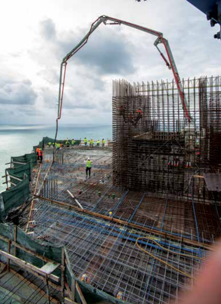
At the Armani/Casa project, FCU proved that a 700-foot vertical push using a truck-mounted pump was not only feasible but extremely effective.
