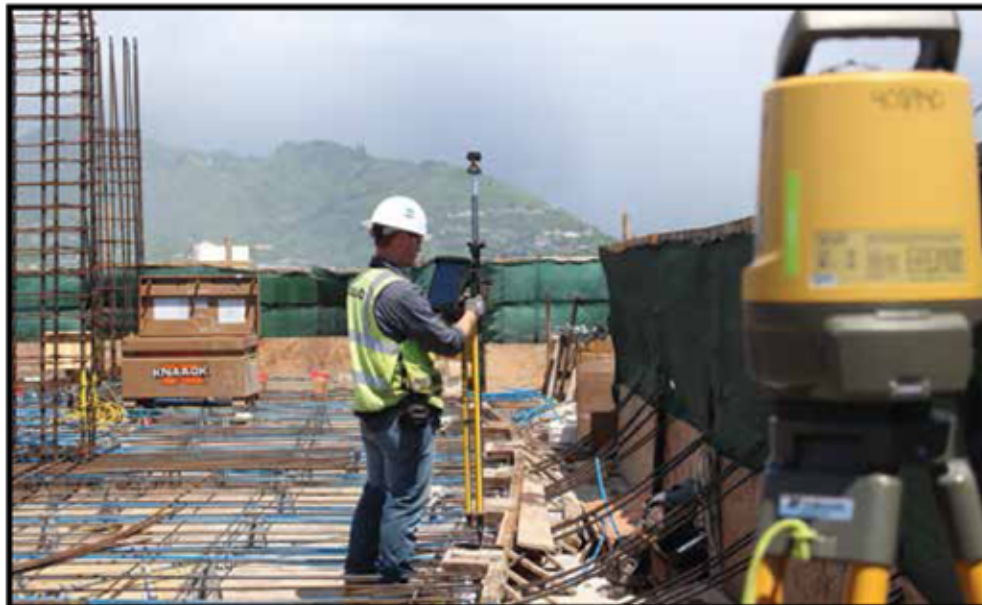
Using the Topcon LN-100, Nordic PCL dramatically streamlined the embed installation process and all but eliminated re-work costs.
